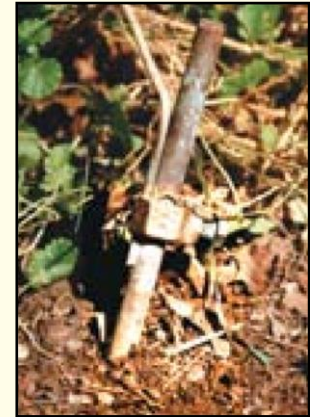
Grounding rod in the earth.
