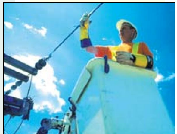
Electrical line workers need special training and equipment to work safely.
