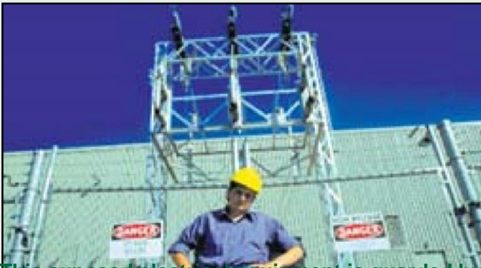
This exposed electrical equipment is guarded by an 8-foot fence.
